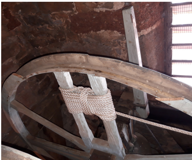
The second wheel with a section of shrouding missing
