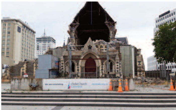
The sorry state of Christchurch Cathedral after the earthquake in 2011 Note the remains of the tower on the left
